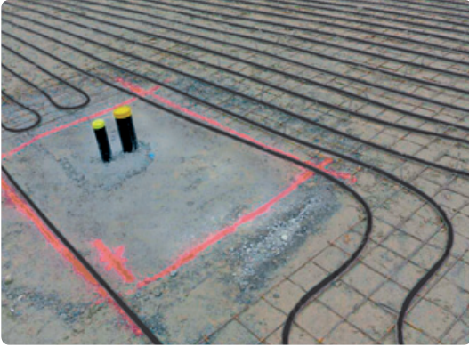
Collector pipe loops made of PE-Xa
