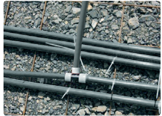
Connection lines made of Uponor ground energy PE-Xa pipes
