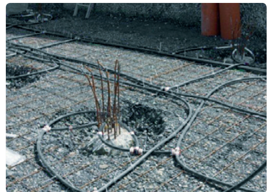
Connection of Energy Piles using Uponor PE-Xa pipes
